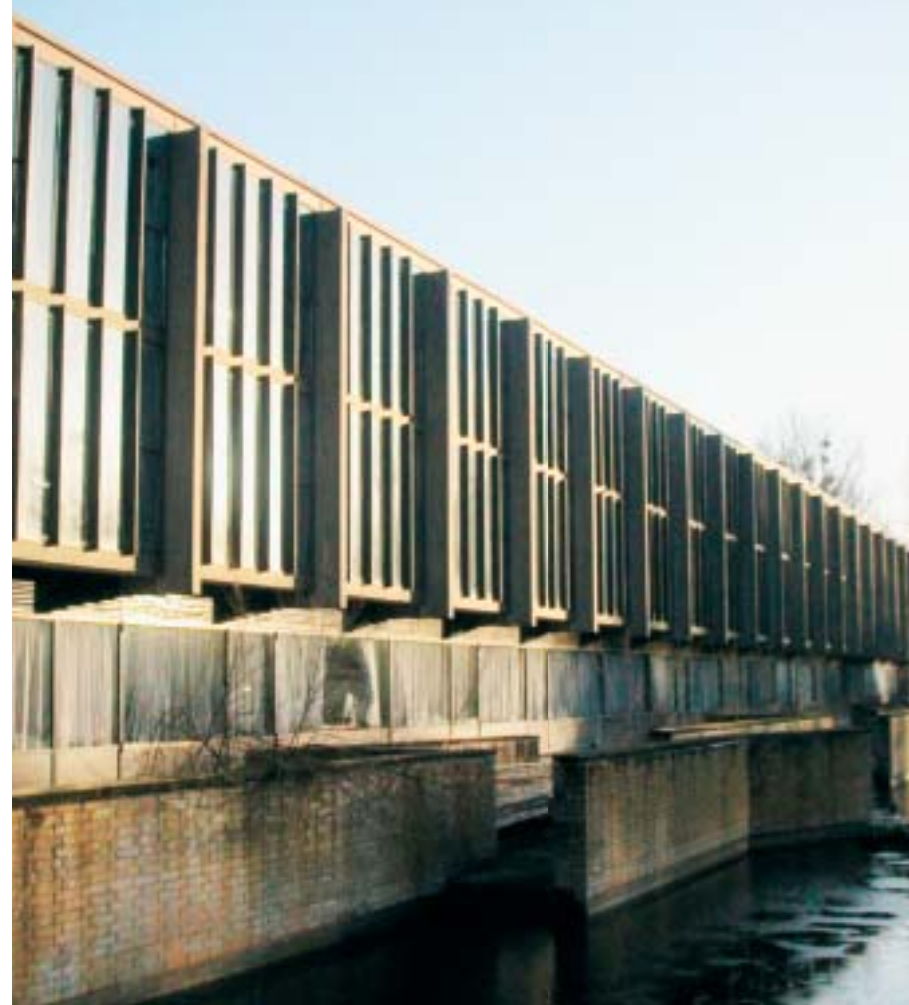
◀ St Catherine's College, Oxford. Image reproduced by kind permission of Allan Haines, The Concrete Centre
